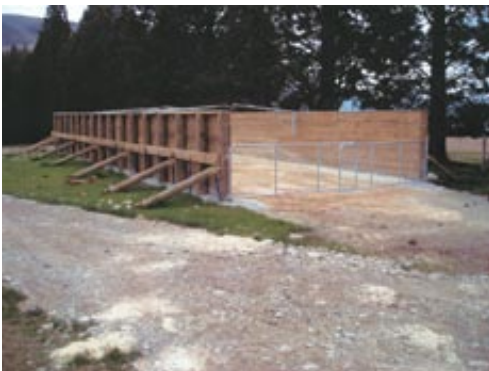
Storage bins and frames for tarpaulin roof
